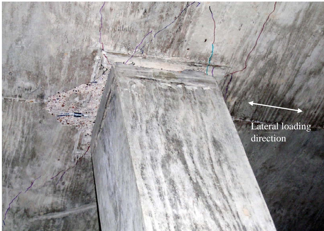
Figure 4.25 Bottom failure surface of L0.5
