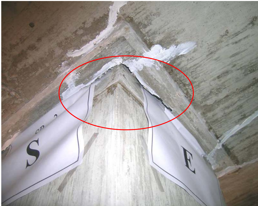
Figure 4.46 Bottom view of failure surface of LRshG0.5
