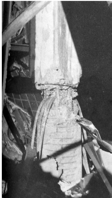
Figure 1.9 Close-up of a slab-column joint at Bullock's Department Store (Mitchell et al. 1995)
