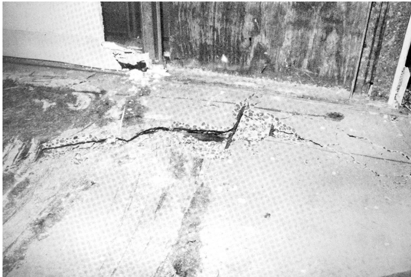
Figure 1.7 Punching shear failure in post-tensioned slab (Mitchell et al. 1990)
