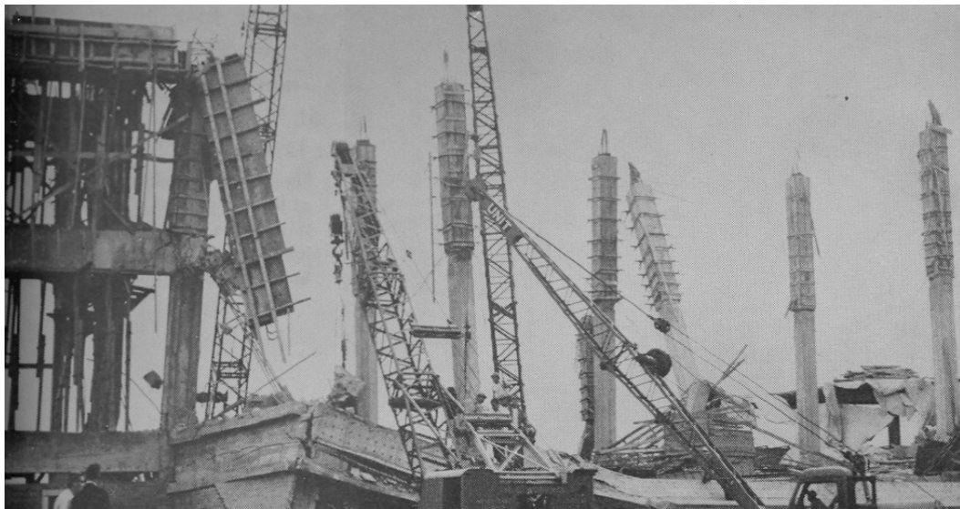
Figure 1.4 Columns remained standing after the progressive collapse (Feld 1964)
