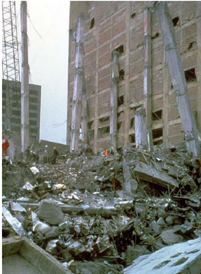
Figure 1.6 Complete collapse of a waffle-flat-plate structure (EERI 1997)
