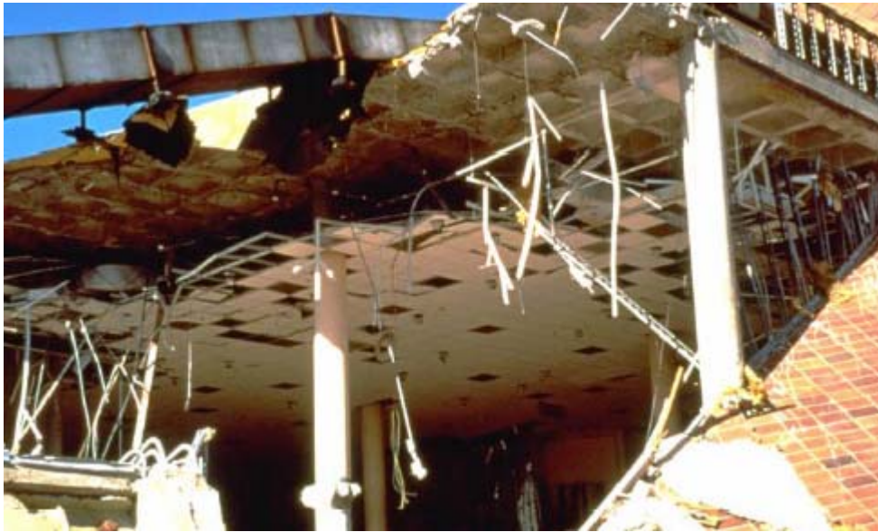
Figure 1.8 Collapse of Bullock's Department Store (EERI 1997)
