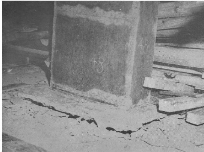
Figure 1.2 Punching shear failure at an interior connection (Feld 1964)
